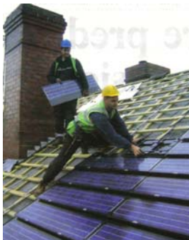
Photovoltaic roof panels
